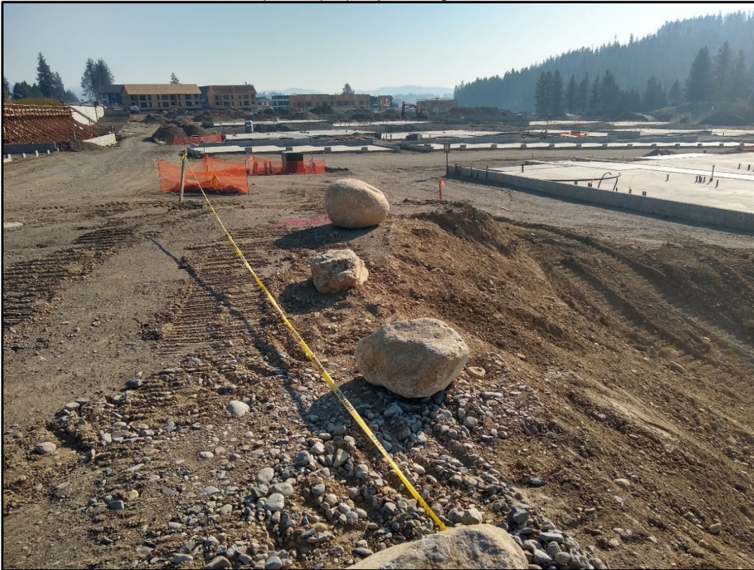
SITE PHOTO - 7: Southeast part of property looking southeast along trail and river.
