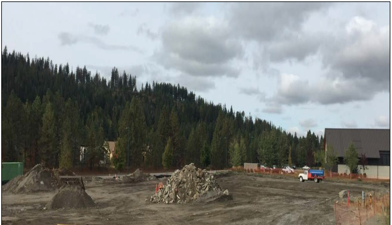
SITE PHOTO - 7: View from the northeast corner of the subject property looking southwest toward the Spokane River and Northwest Bank
