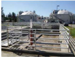
The wastewater treatment plant is taking steps to mitigate visual and odor impacts on its neighbors.
