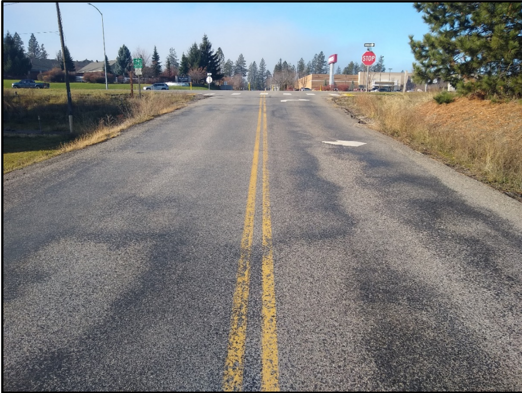
SITE PHOTO - 5: View from the west end of Aqua Avenue looking west.
