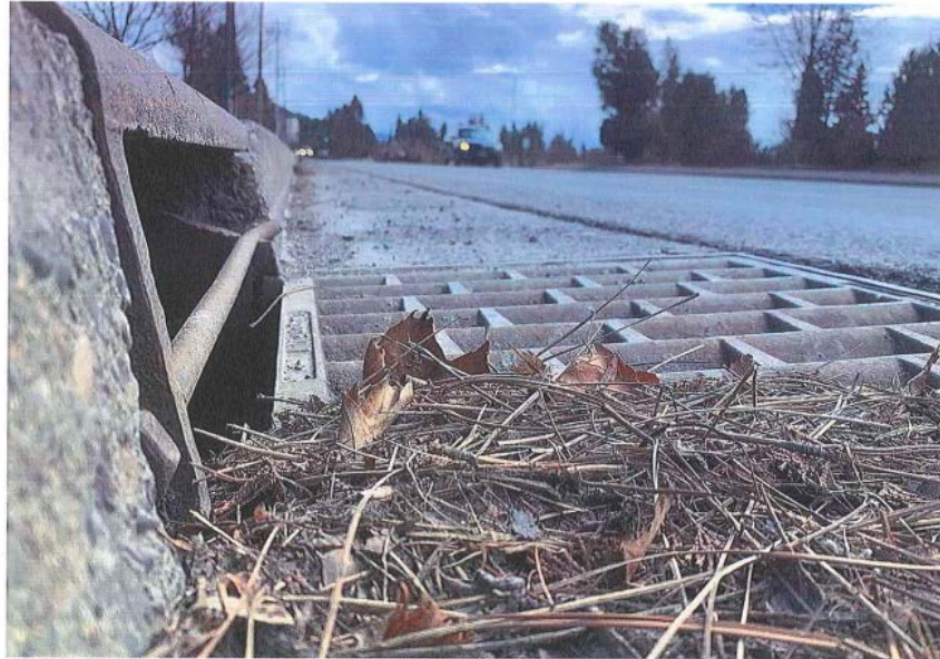
Tree needles rest in the gutter on Northwest Boulevard on Monday. The city of Coeur d'Alene is expected to be clearing Ramsey Road and Northwest Boulevard this week as part of its spring cleanup.
