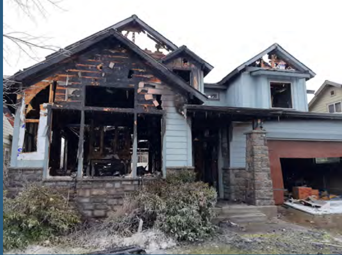
Home damaged by fire Demolition completed January 2022
