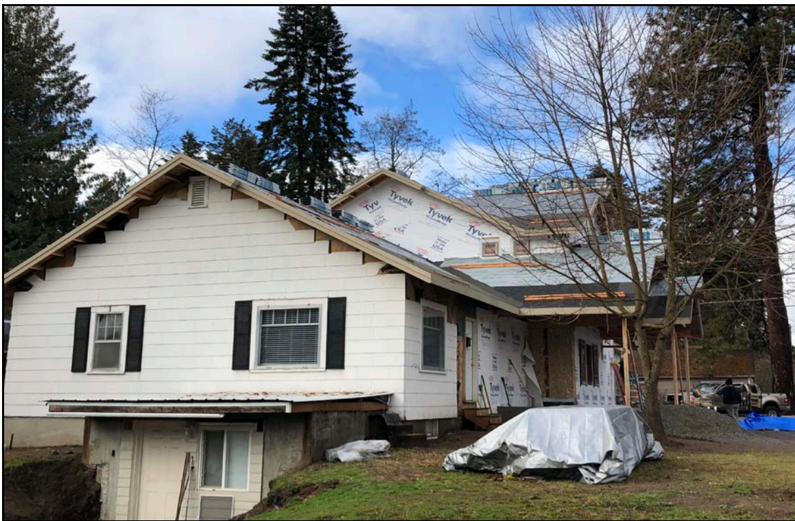
View of the subject property currently under construction, looking west from 14 th Street
